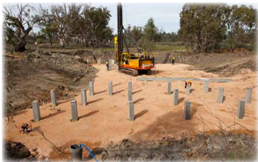
Above: Installation of concrete piles for the Lower Potterwalkagee Regulator, which is replacing the existing Lock 8 Track causeway. Photo: Mallee CMA.
